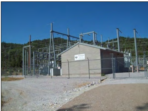
City of Shasta Lake Substation
